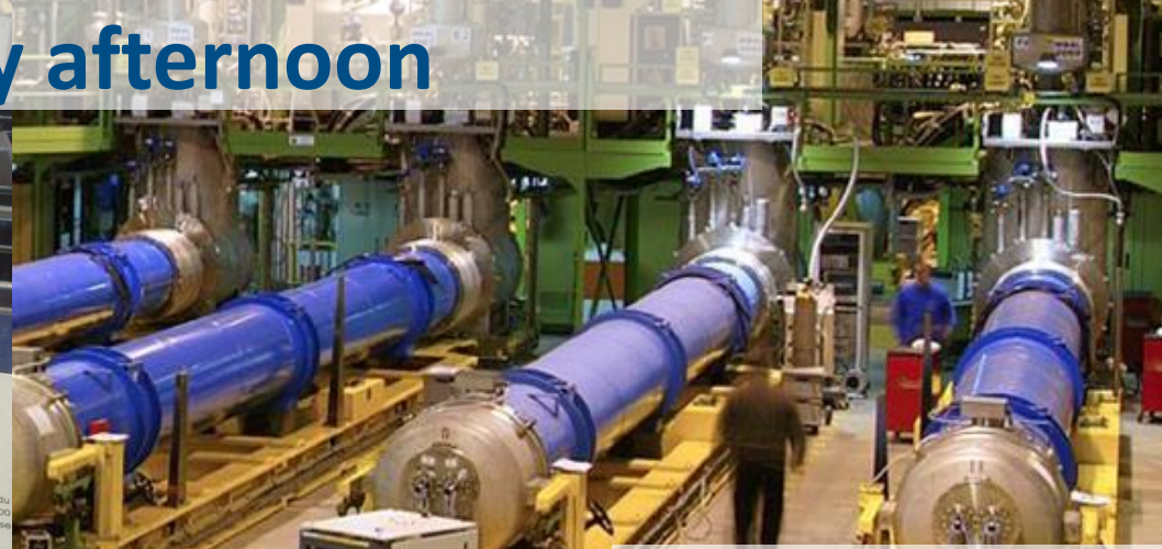
Magnet test facility
