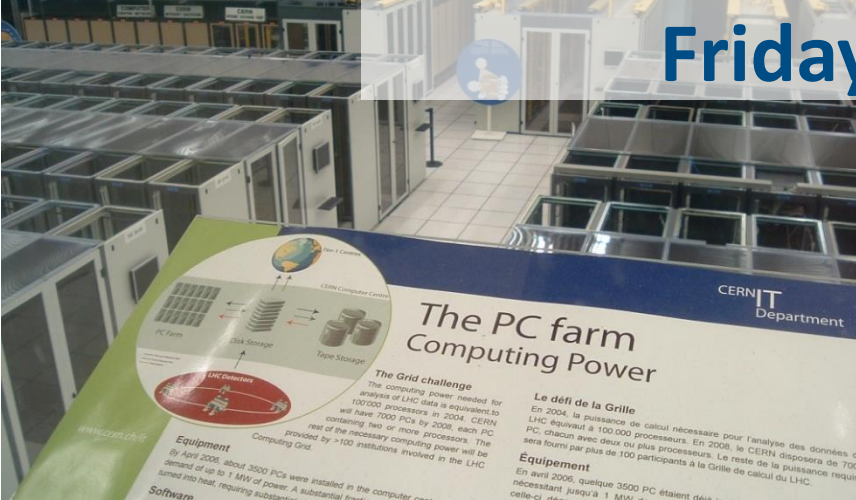
CERN data center
